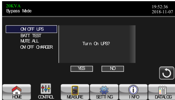
TURN ON UPS
