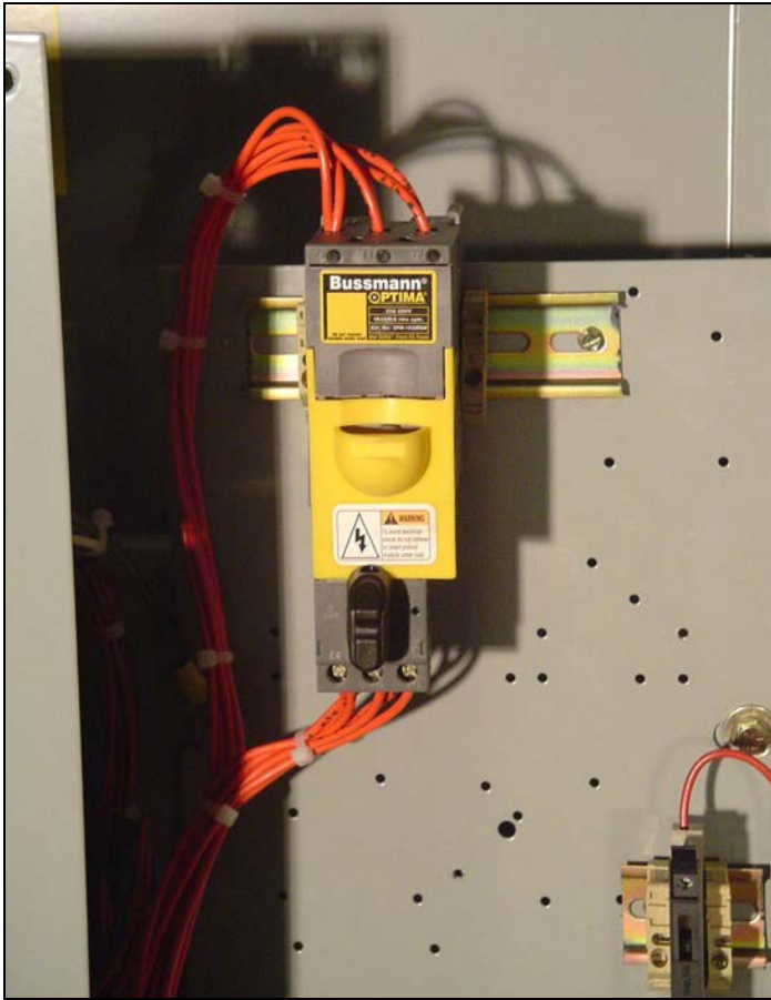
Figure 45. Source 1 Control Disconnect in the ON Position.
