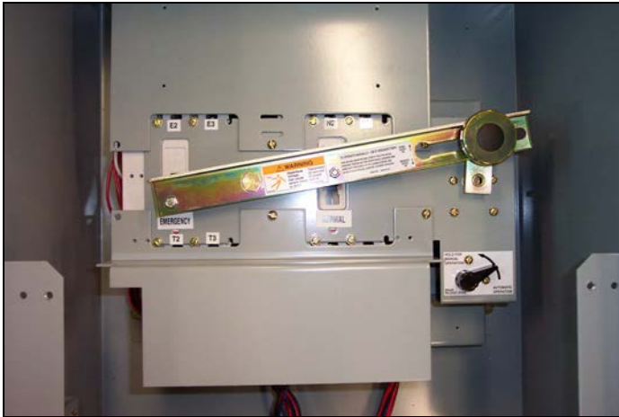
Figure 39. Horizontal Power Panel
