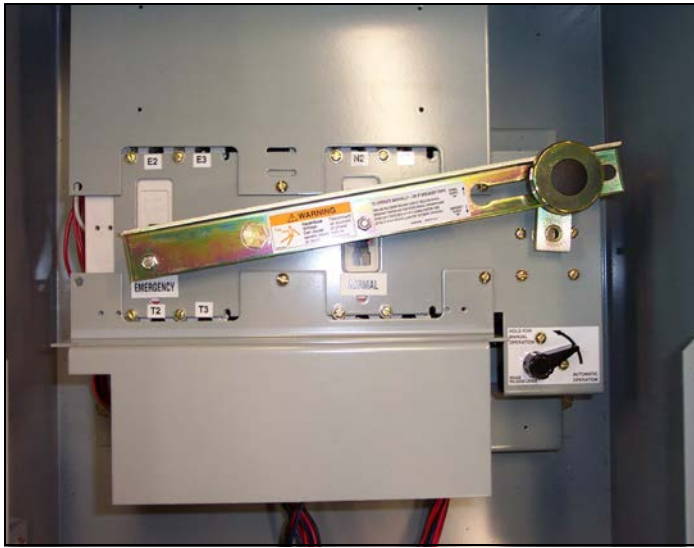
Figure 4. Typical Power Panel for 30-150 A Models (Deadfront Cover Installed).
